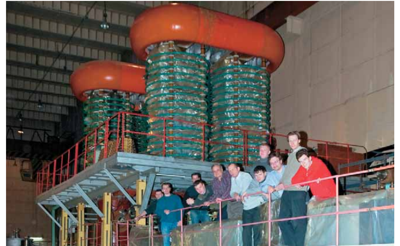
Generator of megavolt pulses of the U-2 accelerator used for plasma heating in the GOL-3 multimirror trap
